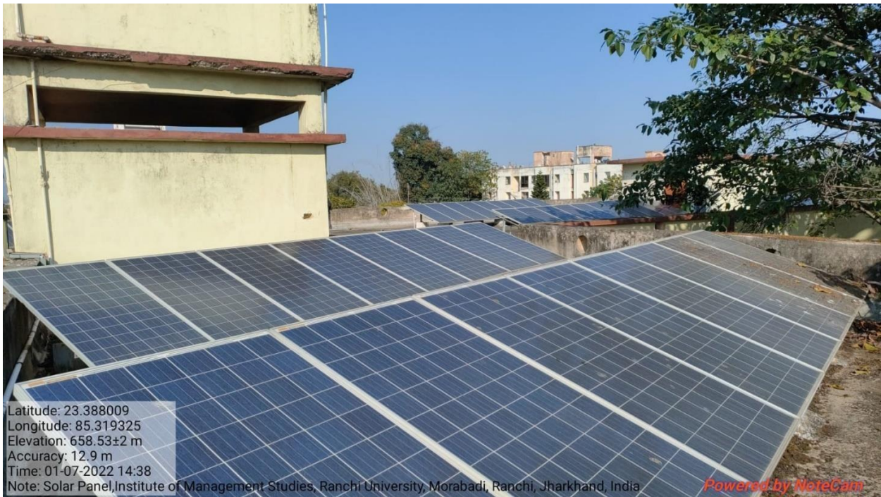
Solar Panels installed within the campuses of Ranchi University
