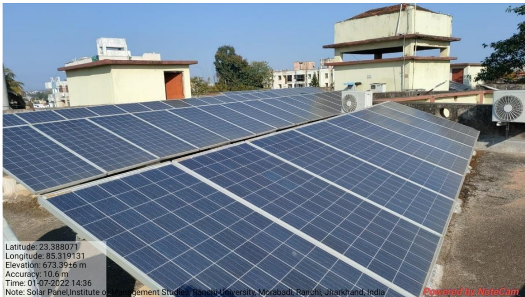
Solar Panel installed at university
